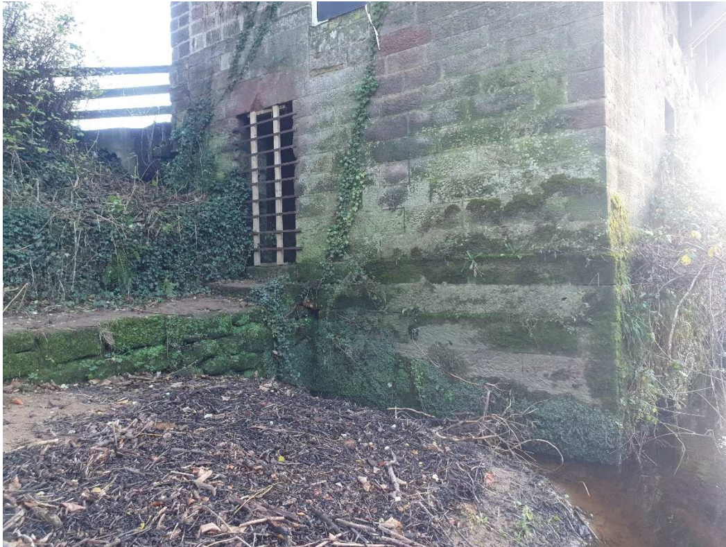
Figure 8: Downstream wall of mill, stone footway, siltation and erosion
